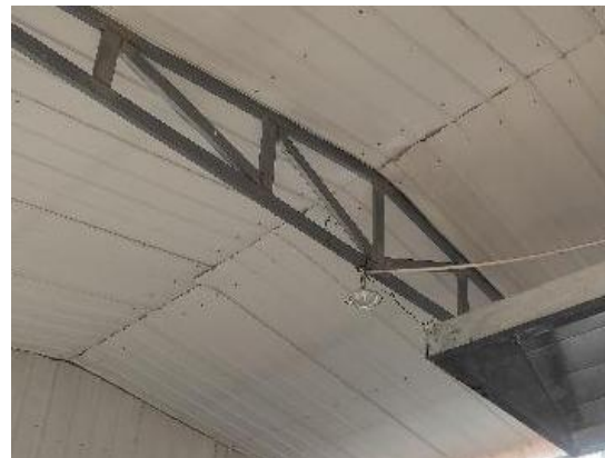
危废库防爆灯
